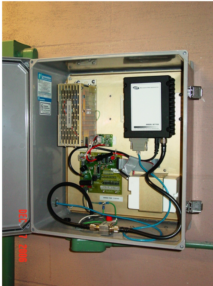
Production Site – Typical Radio Panel
