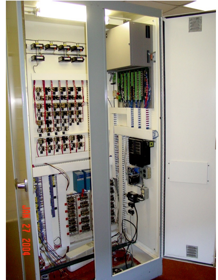
Production Site – Typical SCADA Panel
